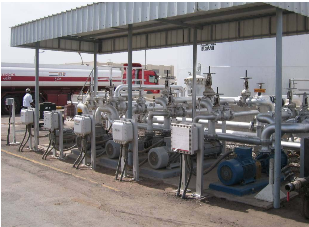
existing aviation fuel pumping station
